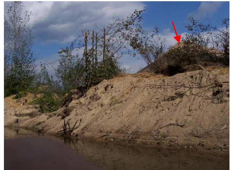
Photograph 16. Temporary spoil piles have been placed above the top of bank (red arrow) and some vegetation replaced, however, sloughing may occur on this site due to exposed steep banks.
