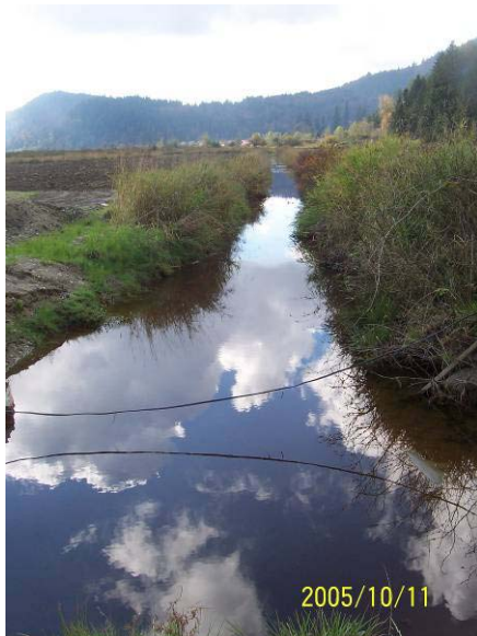
Photograph 22. The Bouchier Creek channel after removal of material from the debris torrent.
