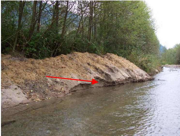
Photograph 13. In a few places, excavator operators placed spoil against newly excavated over steepened banks as they thought it would reduce the grade. During high flow events, this spoil will likely erode.
