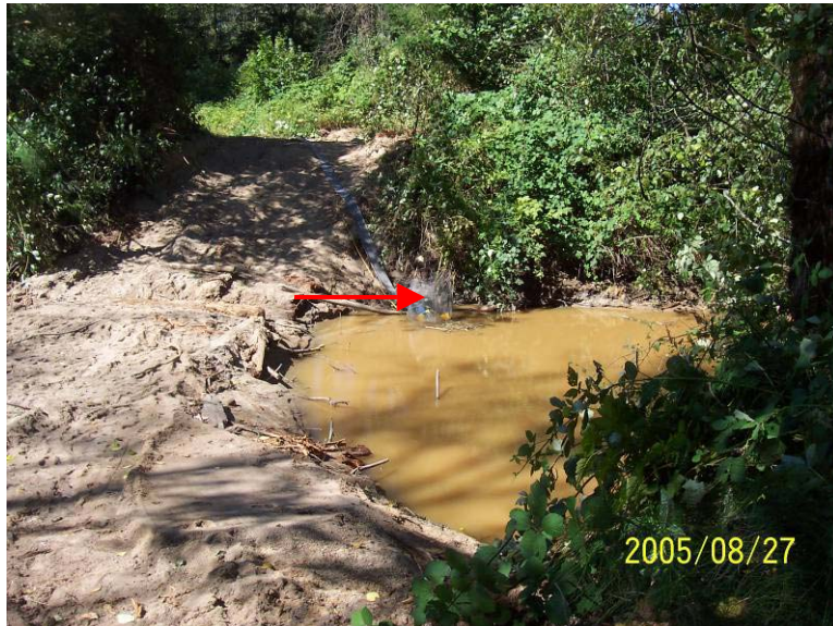
Photograph 9. A substrate berm was constructed approximately 300m upstream from the outlet of the diversion. Silt laden water was periodically pumped into the adjacent forest (red arrow).
