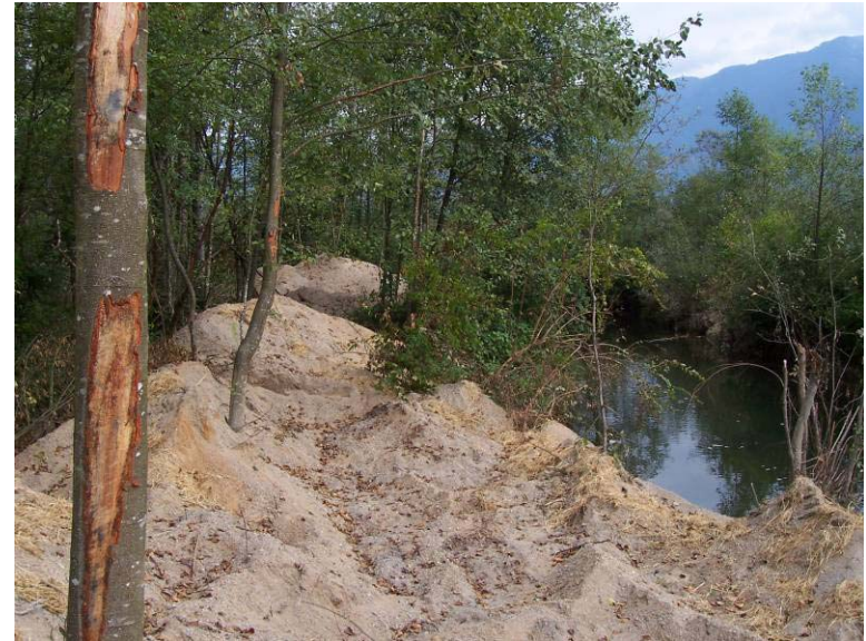
Photograph 15. Looking at spoil piles along the right bank that are inaccessible. Spoil was placed in open spaces, but girdled alder trees. The trees should survive as they will grow advantageous roots.
