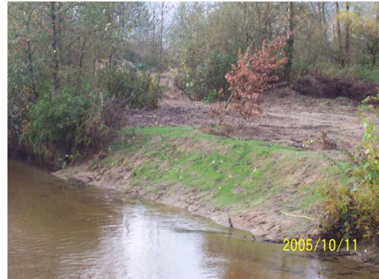
Photograph 15. Looking at the diversion location. Grass seed has taken and no erosion was evident. Beavers had cut some of the planted vegetation and one tree did not survive
