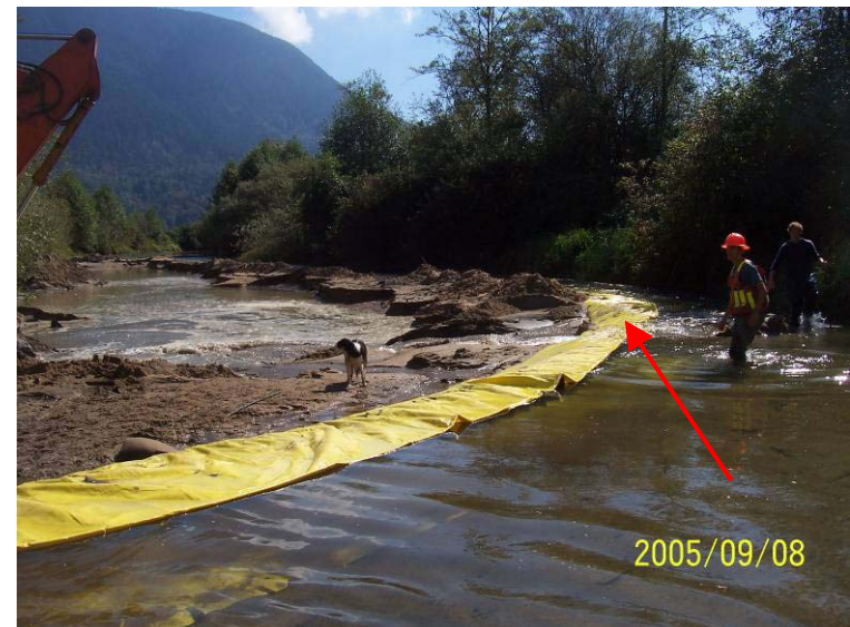
Photograph 8. The Megasecure also failed to isolate flow at the second location. Again, the excavation was almost complete when the failure occurred.
