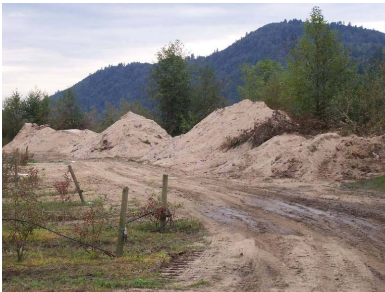
Photograph 14. View of temporary spoil piles on the east side of Lagace Creek. The piles are located behind a small riparian buffer (3 to 5m). Spoil should be removed as soon as possible.
