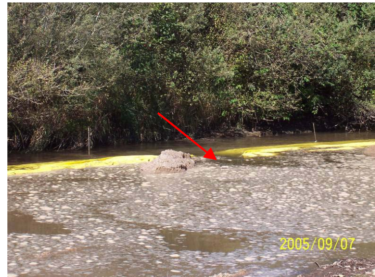
Photograph 7. The Megasecure failed to isolate flow at the first location (water undermined substrate under the Megasecure). Excavation was almost complete when the failure occurred.
